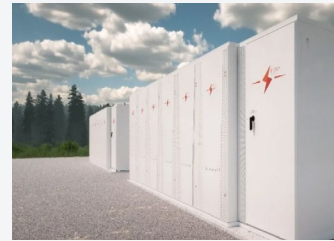
Battery storage area
