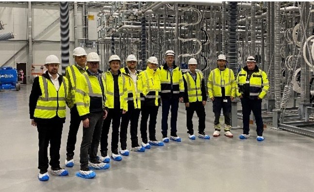
The picture shows an example of a joint safety walk with our customer at our installation site of Viking Link HVDC interconnector in Revsing close to Vejen in Denmark.
